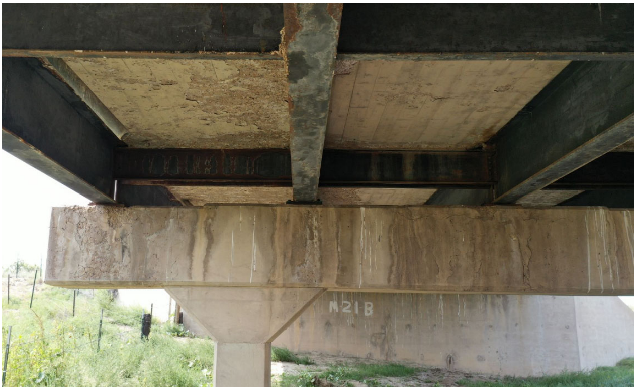
Picture 3 - Corrosion, cracking, efflorescence
